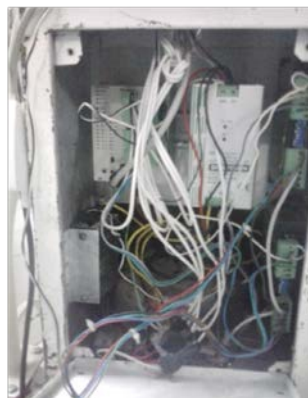
Figure 11. Rear view of stepper motor PLC control unit.
