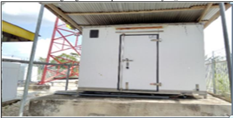
Figure 3: Picture of the Shelter in Ejisu_1 Cell Site
