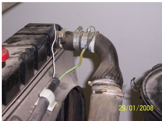
Figure 7: Inlet Radiator Temperature sensor
