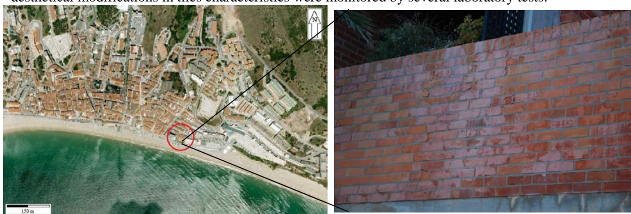
Figure 1 - Aspects of clay bricks degradation due to sea spray action, Sesimbra, Portugal.
