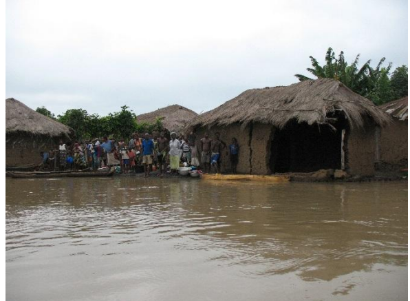
Photo 2 : house partially destroyed (falling) at Ahoho Prise de vue : AFFO, 2016
