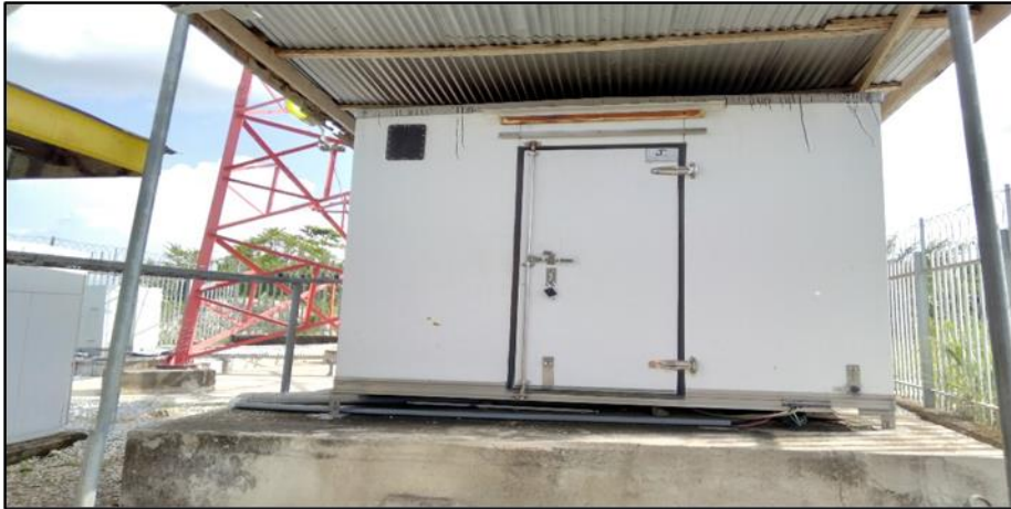
Figure 3: Shelter in Ejisu_1 Cell Site
