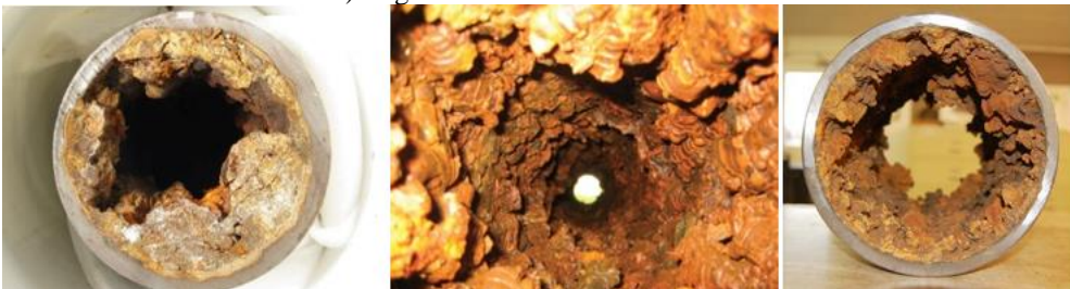
b) Deposits of non-soluble corrosion products (sludge)
