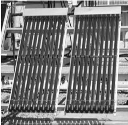
Figure 2: A picture showing evacuated tube collectors used for underfloor heating.
