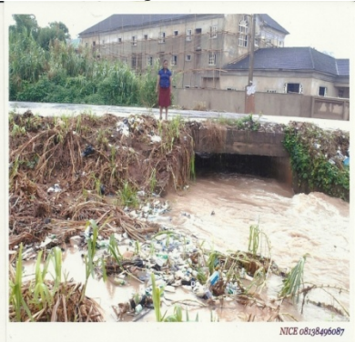
Flooded structures close to the river
