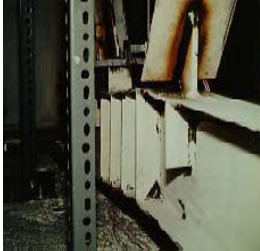
Fig. 8 Large shear deformations in link beam which shape it like a parallelogram
