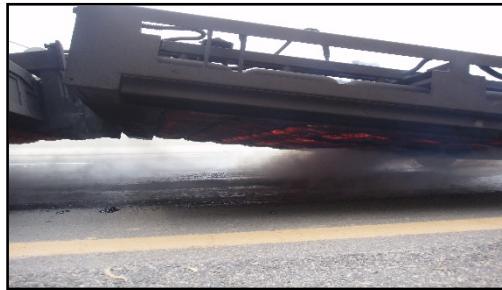
Figure- 5 Pre-heating unit
