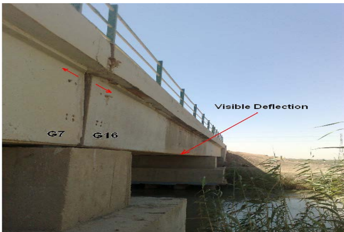
Fig 1 Visible mid span Deflection of the Intermediate Panel
