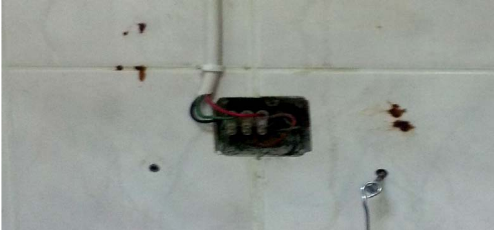
Figure- 17(a): Improper electrical output source.
