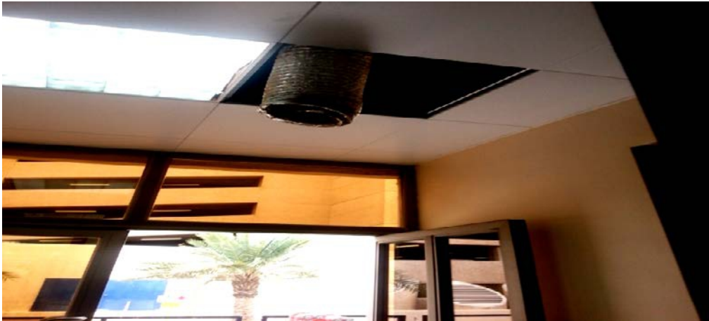
Figure- 16(a): Broken air conditioner.
