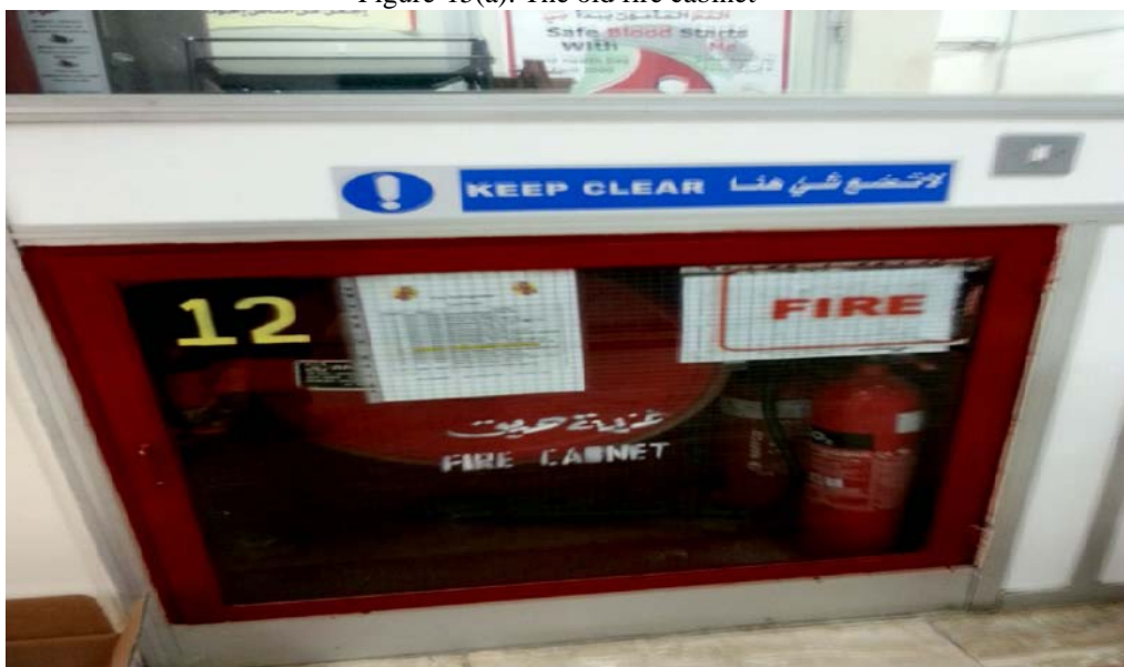
Figure- 15(b): The Recomanded Fire cabinet.
