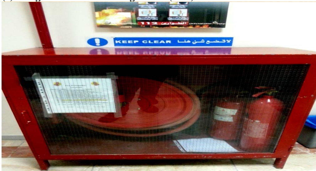
Figure-15(a): The old fire cabinet
