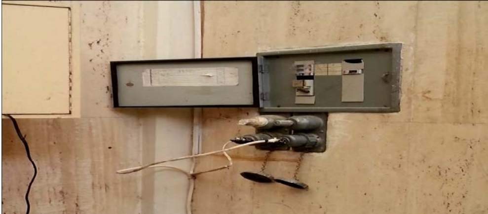
Figure- 17(c): Exposed electrical box in KCBB.
